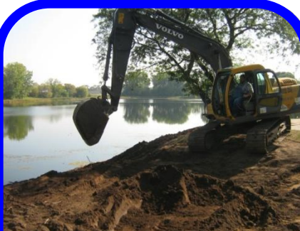
Construction of earthen dike to direct water to slope drain and decrease erosion
