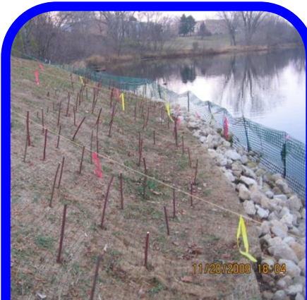
Bank reconstruction area after seeding, stabilization with erosion control blanket, and installation of dogwood stakes.
