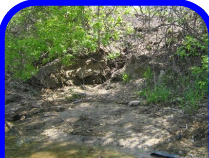
View of gully erosion on bank due to concentrated flow
